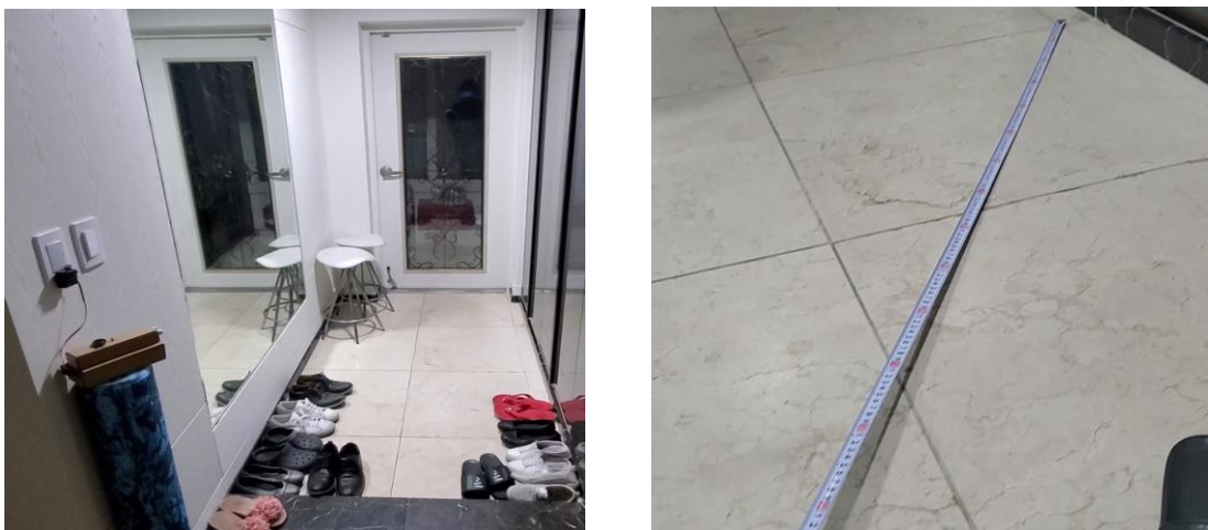
Figure 2: This is a photo of wide view of installed trespassing alarm security system (left). Also, it is important to measure the exact distance to the wall from the sensor to avoid the sensor detecting the wall as a person. So, I measured this distance for my house's front door and set it as a maximum distance in the arduino code.
