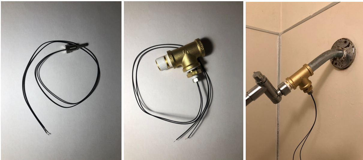
[Figure 3]: From left to right, the thermistor alone, installed in plumbing adapters, and, finally, put in line with the shower head.
